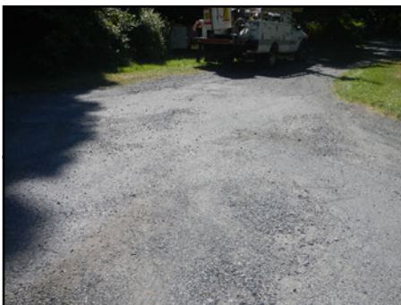
Asphalt deteriorated - appears gravel.
