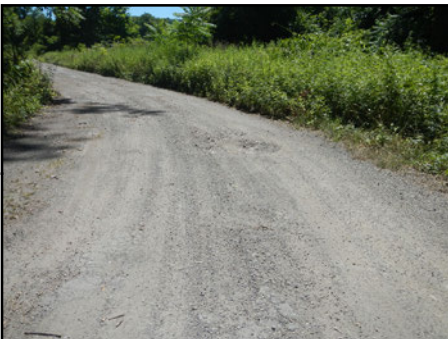
Asphalt deteriorated - appears gravel
