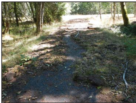
Campground area was not rated due to severe washed out in the area.
